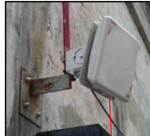
RFID Reader adjacent to Weight-bridge
