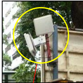
RFID Readers for Trucks entering & leaving the Site
